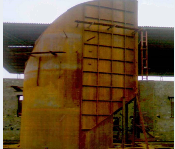
Pre-Heater gas duct
