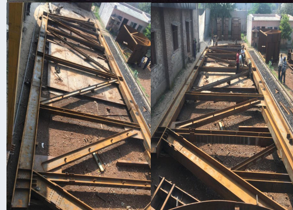
Prilling Tower truss assembly for Project : Chambal Fertilizers and chemicals limited , Kota Weight : 300 MT
